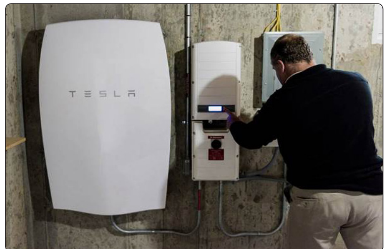
Home battery storage, like the Tesla Powerwall, is now available from area solar installers.
