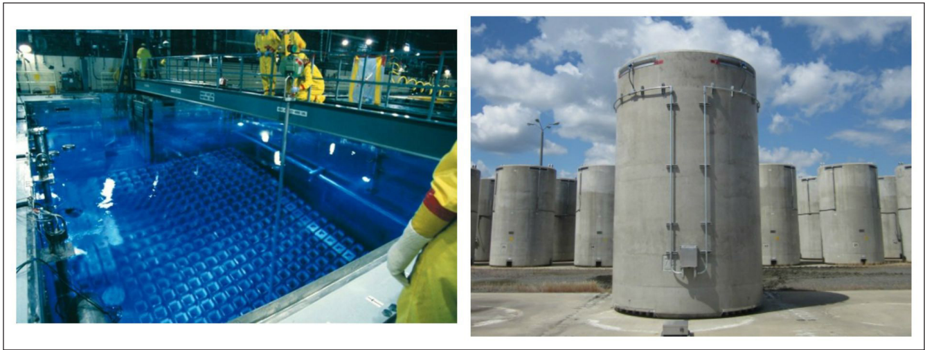
Figure 3. Used Radioactive Fuel Pool and Used Radioactive Fuel Dry Casks 31
